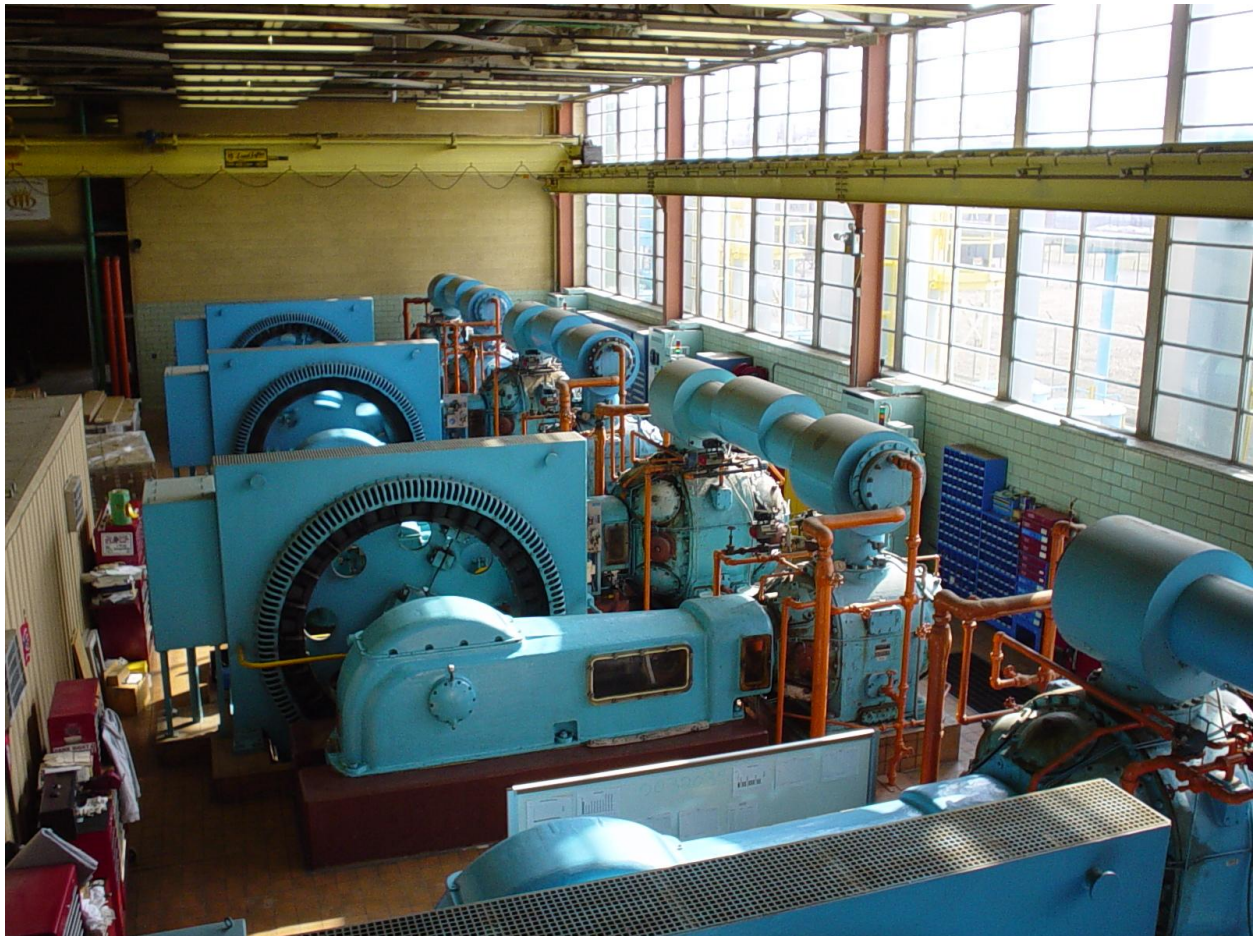
Photograph 1 These reciprocating compressors are powered by 1,000 hp synchronous drive motors. These reciprocating compressors are not considered oil-free, they can be near oil free and capable of reducing oil consumption by retrofitting to carbon-impregnated Teflon piston rings and Teflon wear bands. Each of these units only consumed one- gallon of oil per day. Any oil that is carried over is removed from the air by 0.01 Micron coalescing filters on the compressor discharge which remove 99.5% of the oil, making them virtually oil-free.
